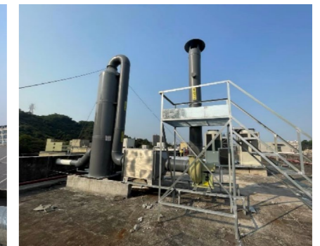
Spray Tower Waste Gas Treatment Facility
